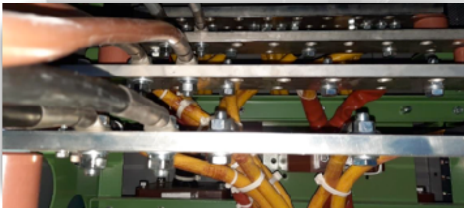
Electrical connections at main generators
