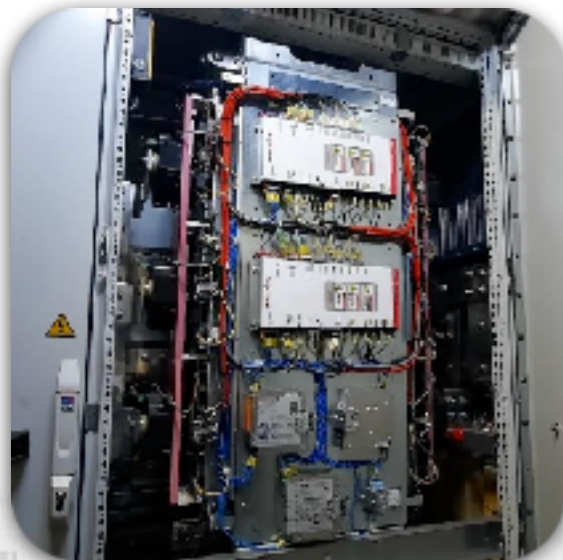
Drive motor variator panels
