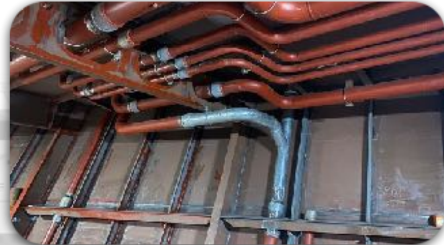
fire fighting system & tanks vents
