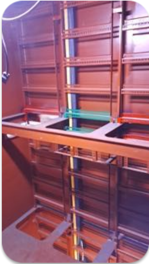
Main wiring trunk (from labs deck to bridge)
